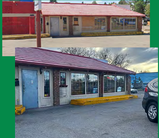
Before, broken and boarded windows at Shepe's Bar. After, plywood down and repairs made.
