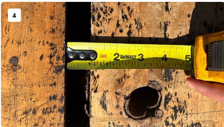
Gaps larger than 1/4" - Needs new decking to meet manufacture spec.
