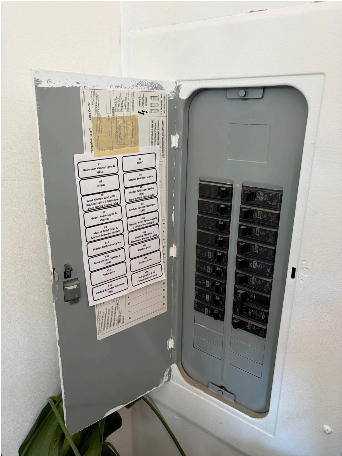
Completed Electrical Hook Up (photo 4)
