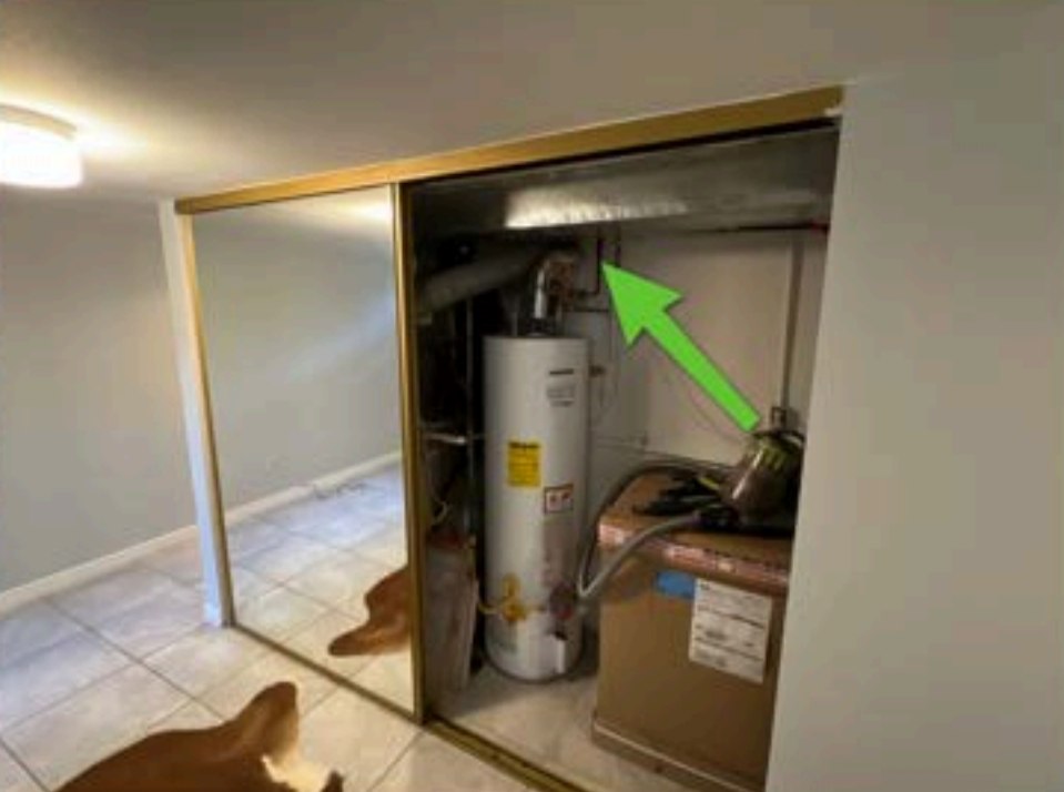
35. Water heater location (disregard green arrow)
