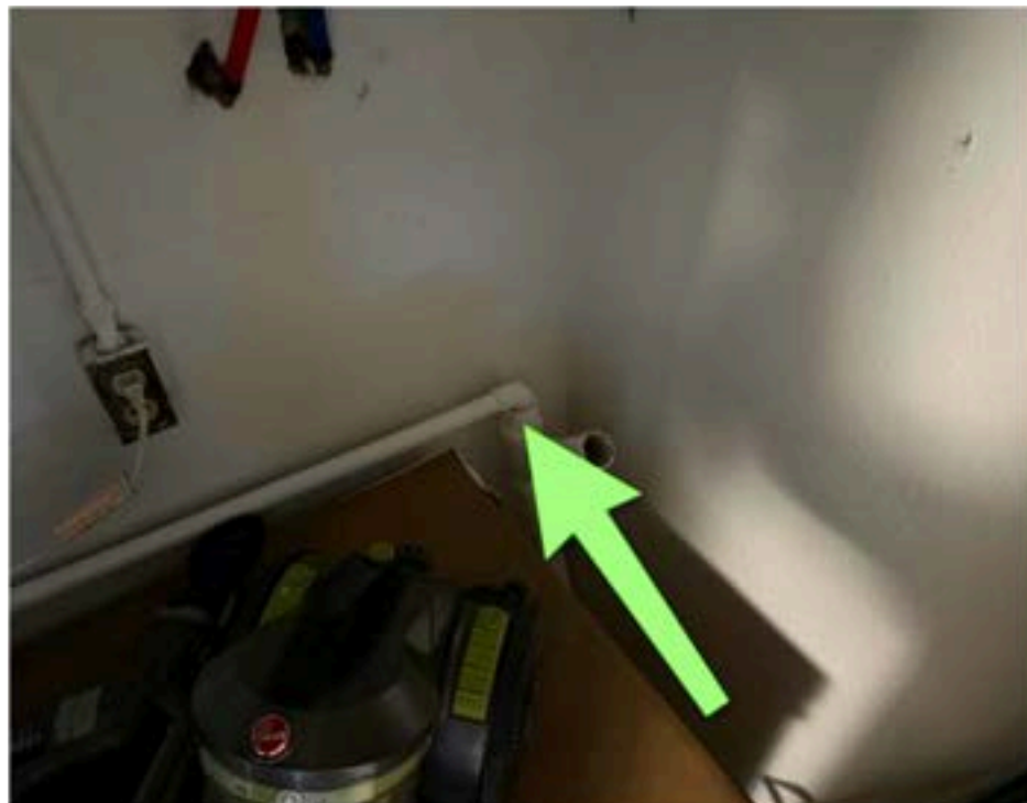
18. Condensate drain (located near furnace)
