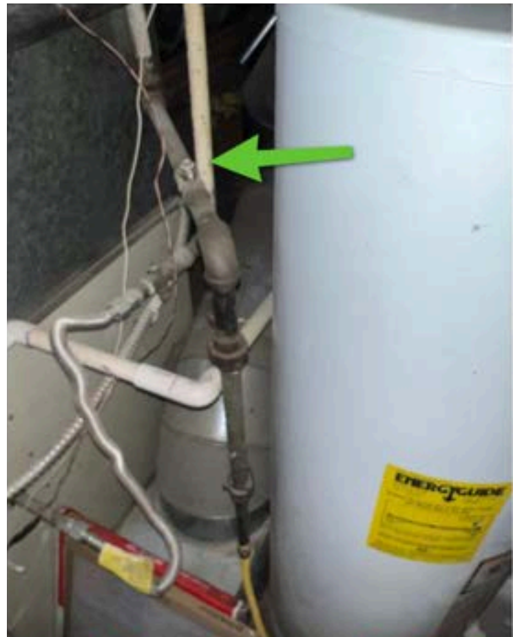
37. Water Heater gas shut off
