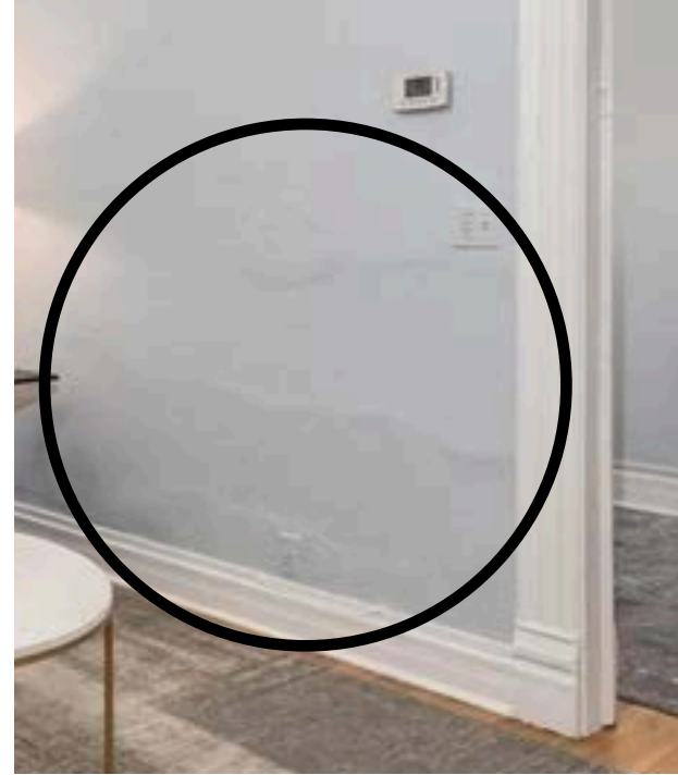
39. Cracking plaster on north wall of living room
