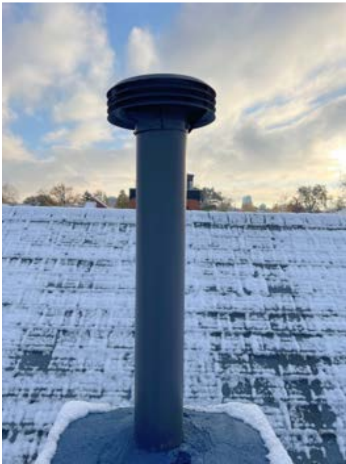
27. Flue Vent pipe on roof
