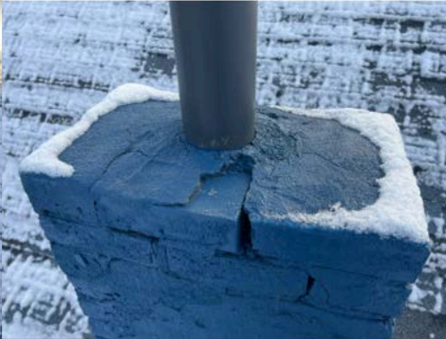
28. Crowned cap and masonry defect on chimney
