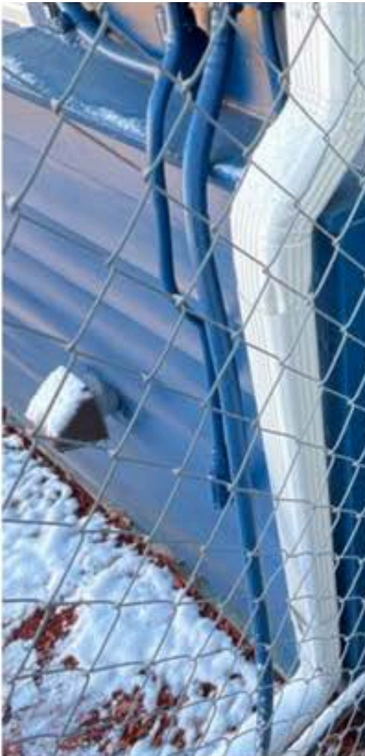
16. Refrigerant lines- Suction & Liquid lines
