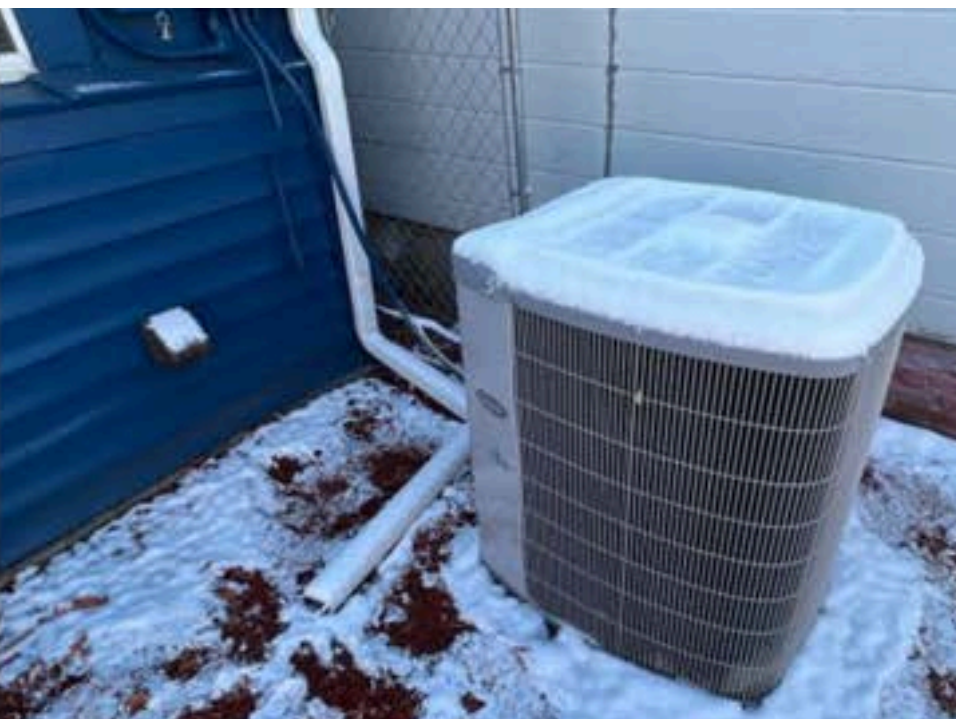
14. AC unit & service disconnect
