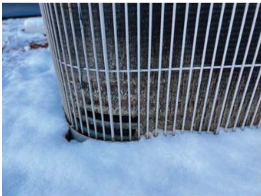
13. Visible corrosion on AC unit
