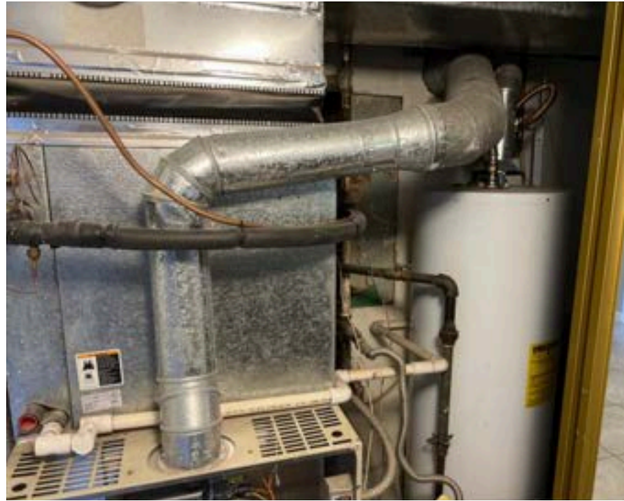
20. Single wall flue venting
