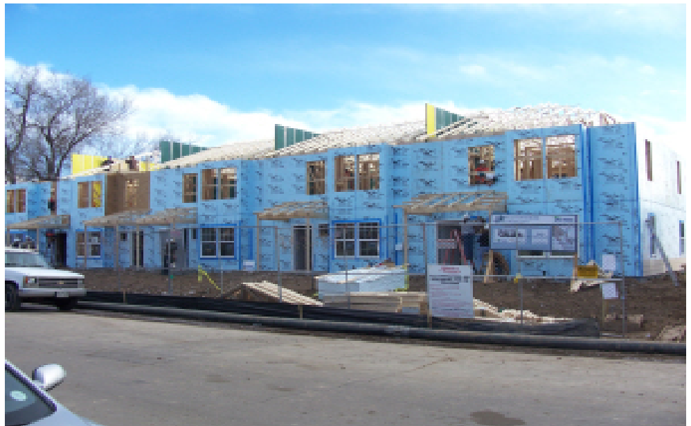
Habitat for Humanity's new 24-unit townhome project is going up in the Virginia Village area south of Interstate 25 and east of South Colorado Boulevard.
