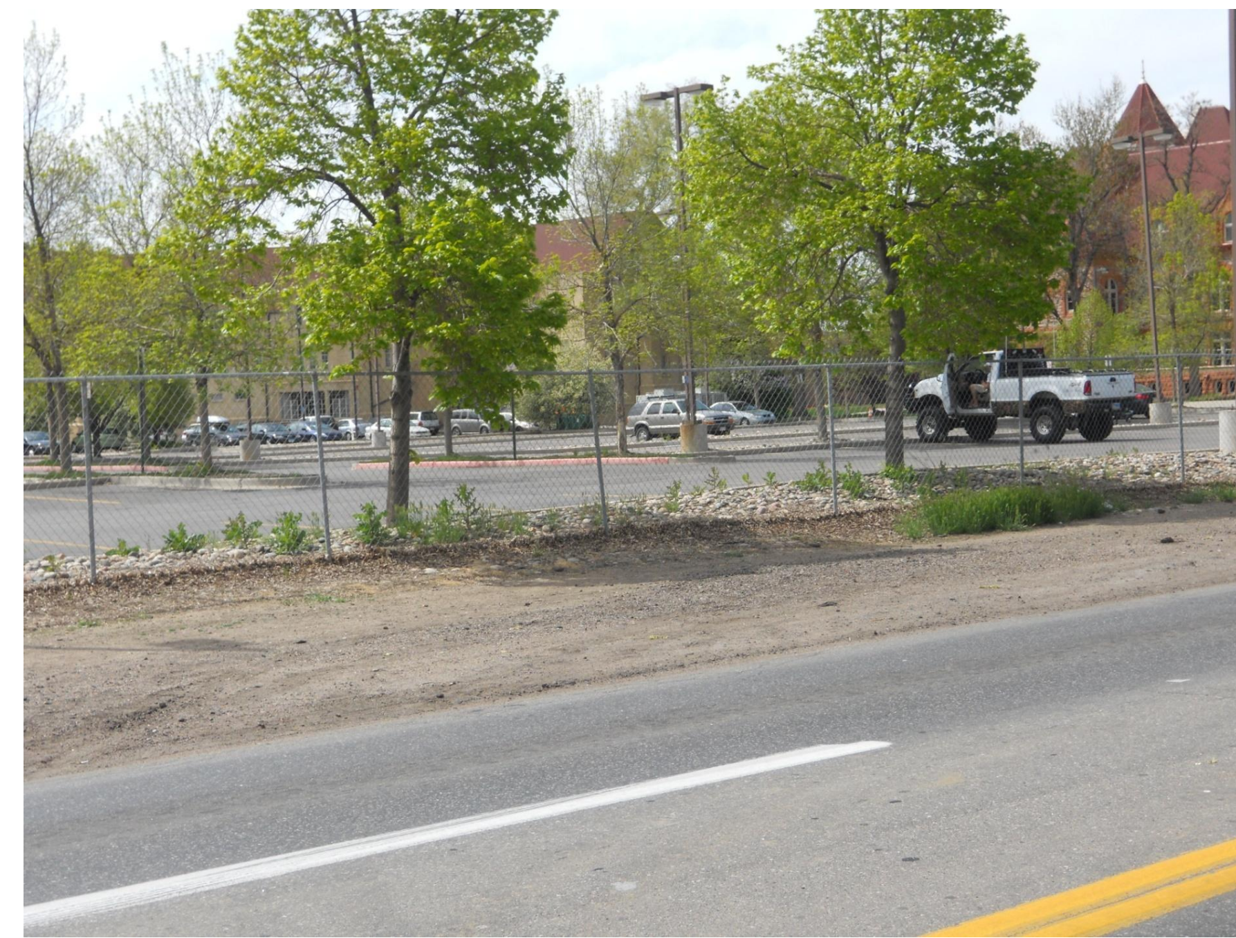
Lack of Roadside Drainage on Quebec St along Johnson & Wales University
