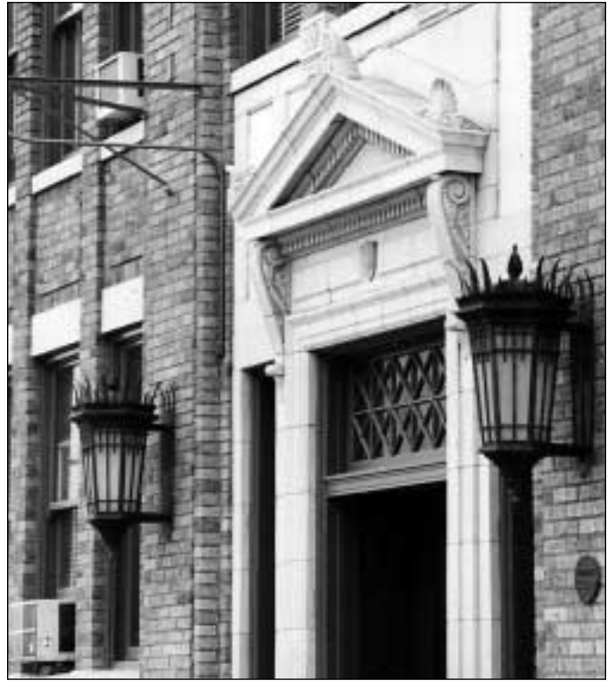
If added entry illumination were called for in the rehabilitation of this landmark building, new or added sources could be accommodated in the generous original lanterns.
