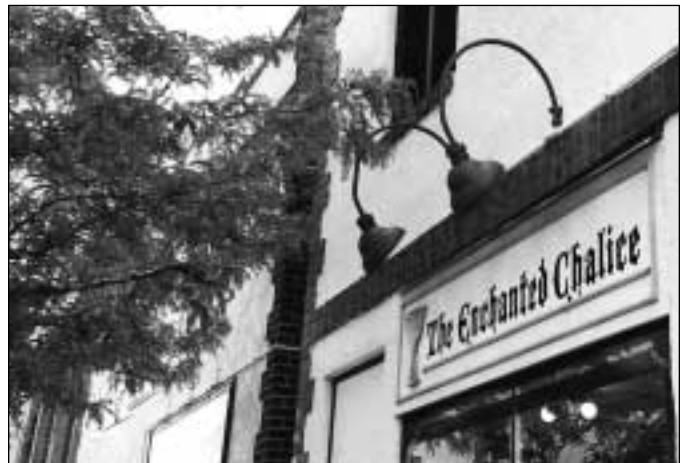
The sign-board fixtures are fed from surface conduit without damage to the brick banding.
