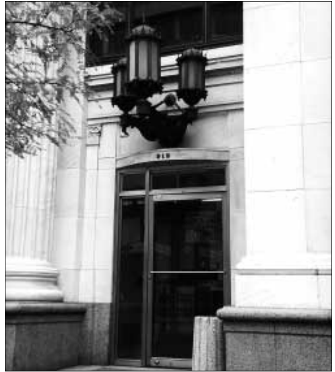
Note the dangling exposed floodlight below the monumental left lantern. Additional down-light to this entry is needed, but could better be achieved with careful modification of the existing historic fixture.
