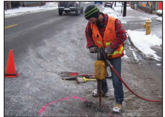
Survey crews excavated existing range points to verify property lines fronting Tennyson Street.
