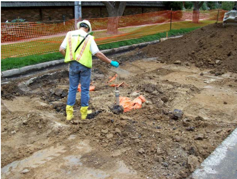
Impacted material uncovered below previous utility trenches.
