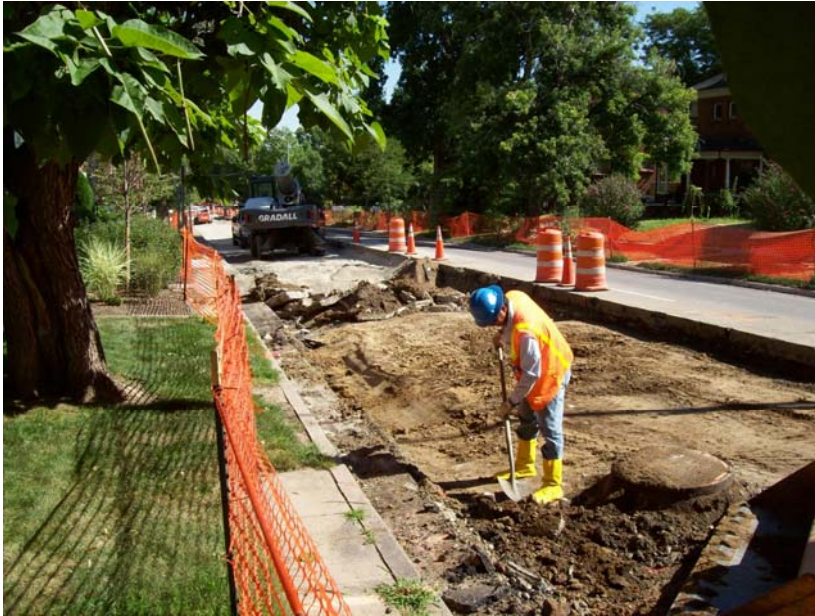
Excavation of impacted asphalt material between 12 th and 11 th avenue on York St.
