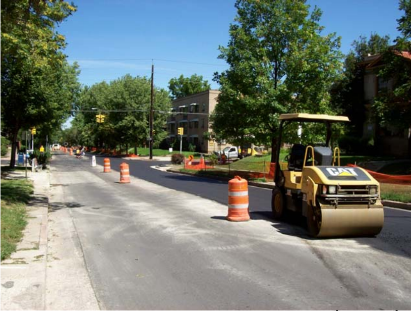
Reconstruction and paving activities between 13 th and 11 th Ave on York St.
