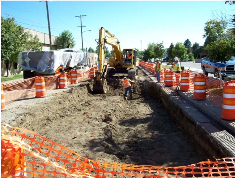
Impacted subgrade delineation in Phase 1 West.
