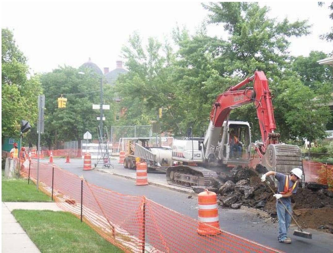
Removal of contaminated asphalt on the east side of Corona Ave. between 7 th Ave. & 8 th Ave.
