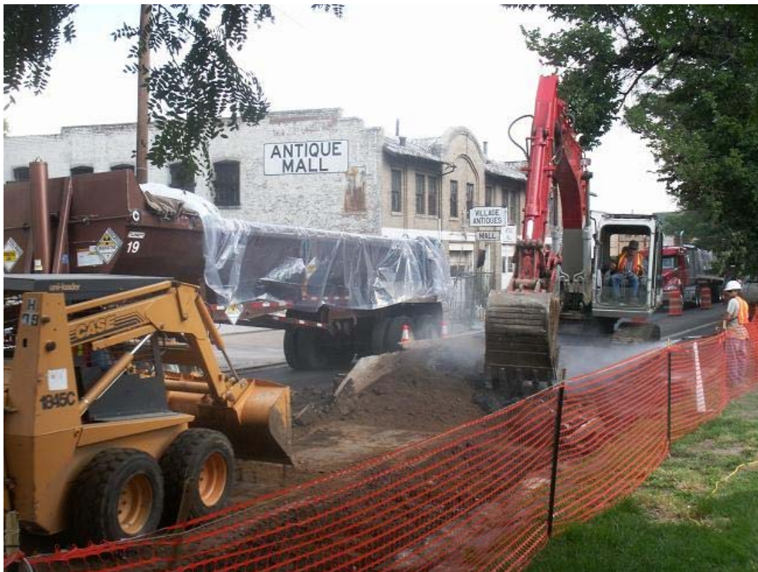
Removal of contaminated asphalt on the east side of Corona St. between 8 th Ave. & 9 th Ave.
