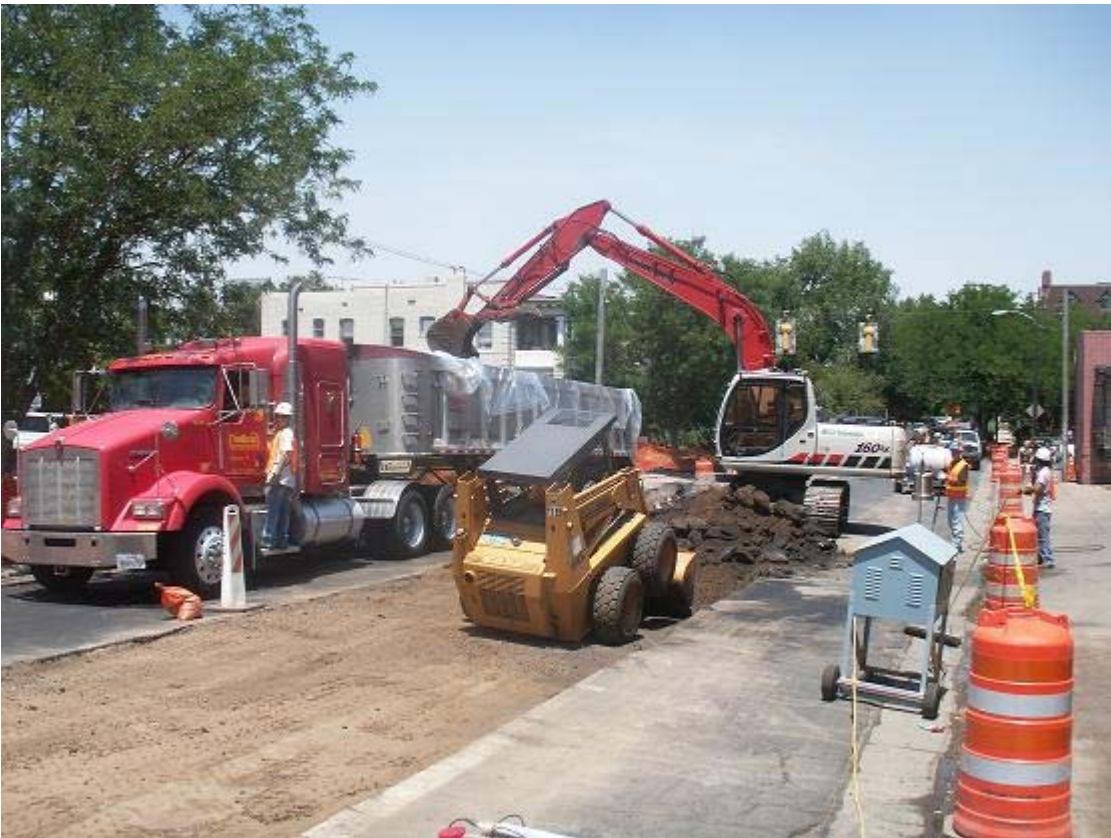
Removal of contaminated asphalt on the east side of Corona Ave. between 9 th Ave. & 10 th Ave.
