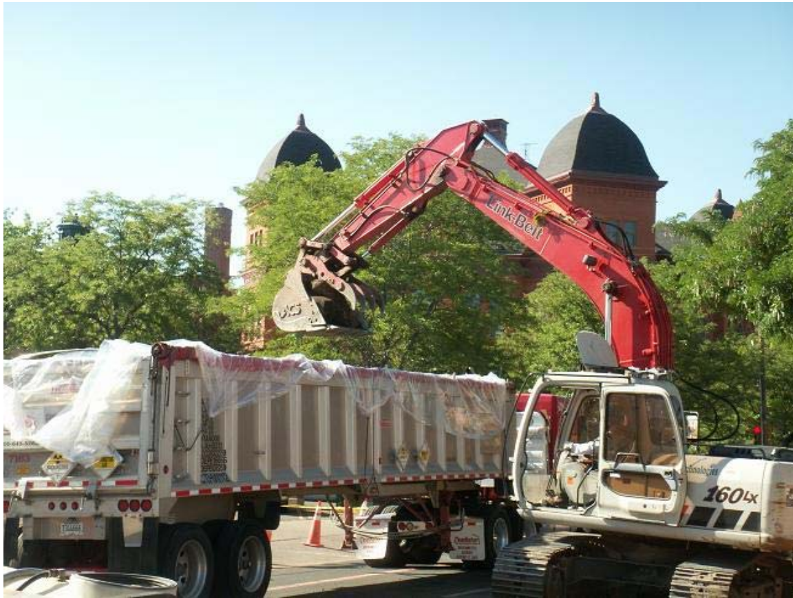
Removal of contaminated asphalt on the west side of Corona Ave. between 9 th Ave. & 10 th Ave.
