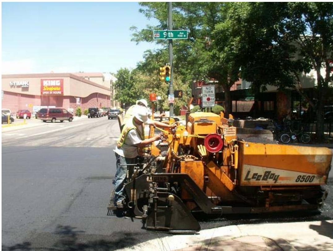
Asphalt paving operations (top lift) on 9 th Ave. from Downing St. to Cheesman St.
