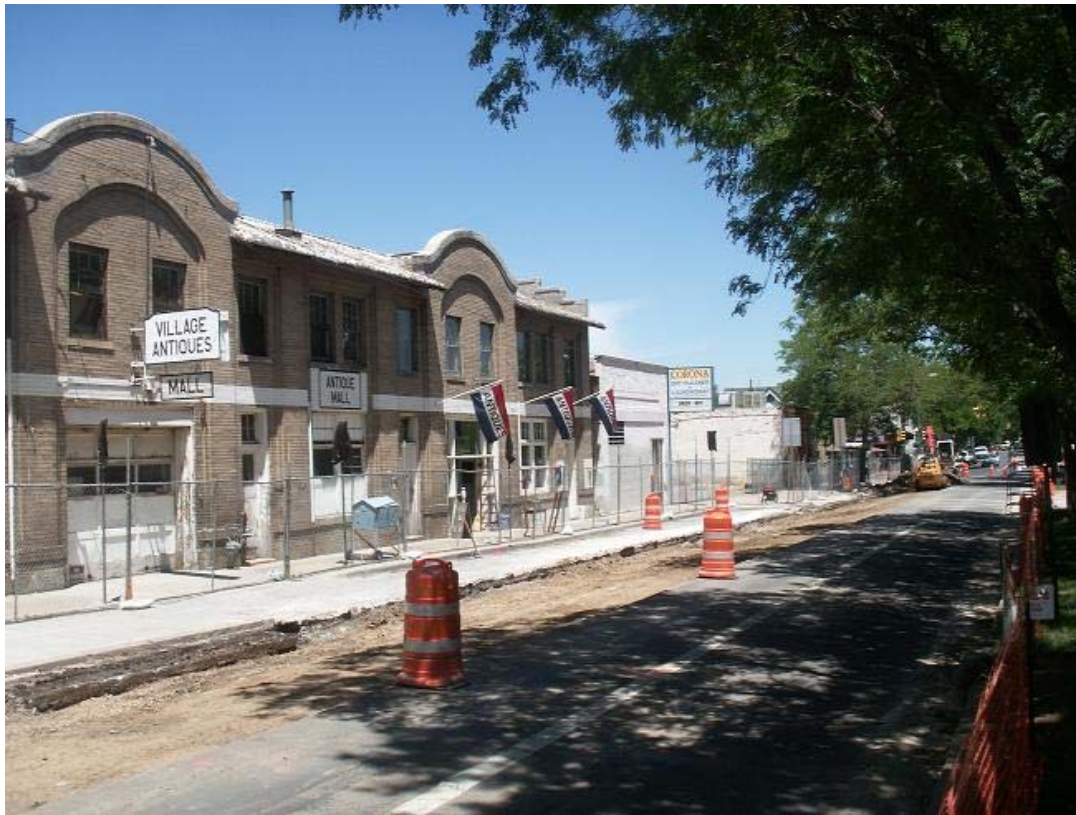
Removal of contaminated asphalt on the west side of Corona St. between 8 th Ave. & 9 th Ave.
