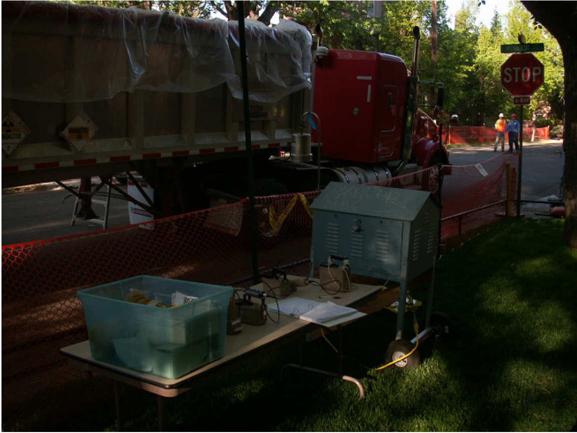
Lined truck bed, air-monitoring system, and hand-held radioactive detection equipment
